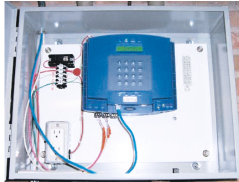
The eBuilding Network Controller, one of nine installed at District 63
